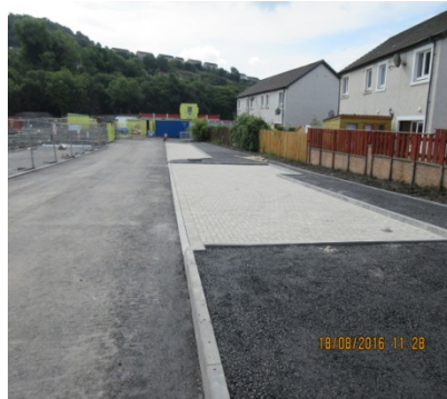
20a New access road and footpath to the rear of McCall Terrace
