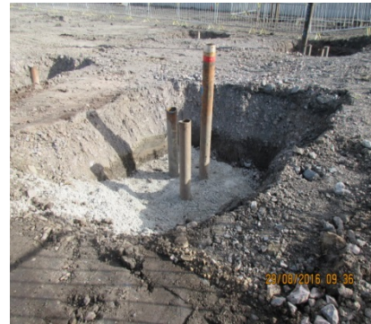
19b Concrete binding laid to enable piles to be cut to correct length
